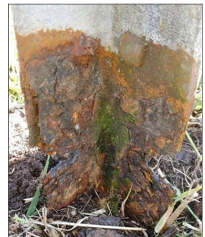
Protection Failure: Unseen underground damage
