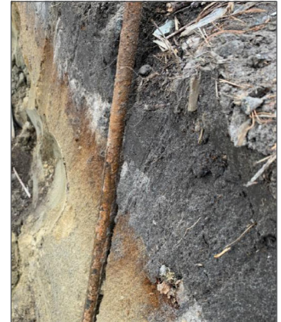
Ground Rod Failure
